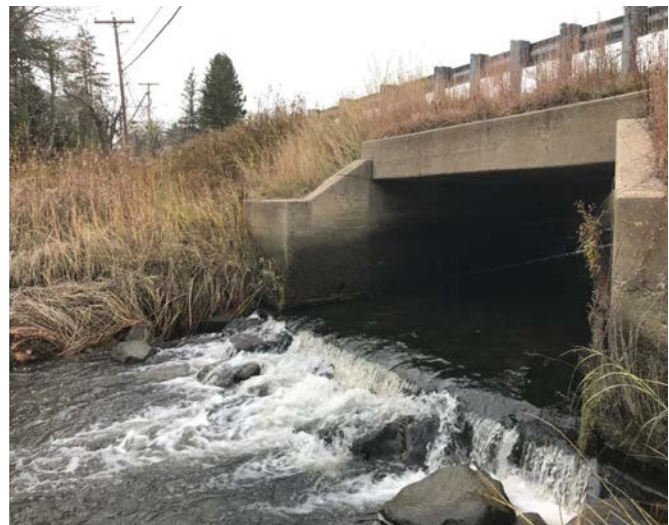
The perched outlet of the Route 91 culvert on Smelt Brook blocks upstream fish passage. Photo: Wells Reserve
