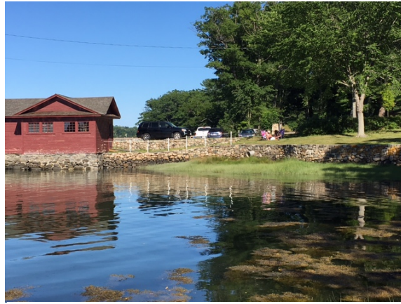
Retaining wall extending from Sewall’s Bridge onto Elizabeth Perkins House property. Photo: Joan LeBlanc
